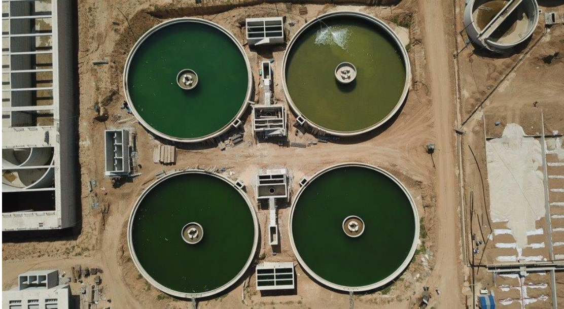
Casted Reinforced Concrete and Water Tightness Test for the Clarifiers in March 2018
