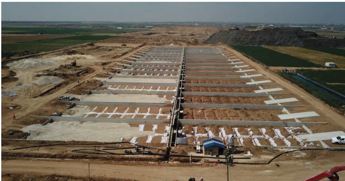
Casted Reinforced Concrete and Installed Perforated Pipes for the Drying Beds in March 2018
